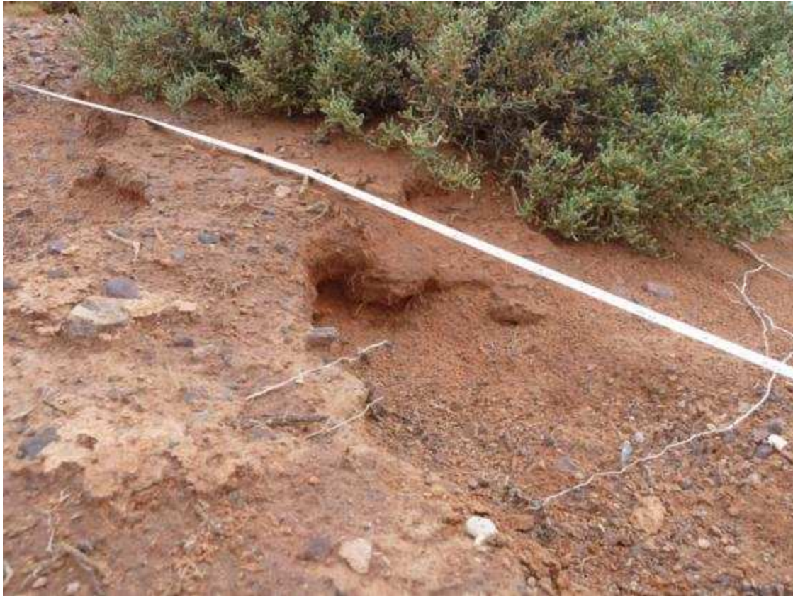
Above and Below: active erosion occurring along the LFA transect within the fenced area at Wurldunda.
